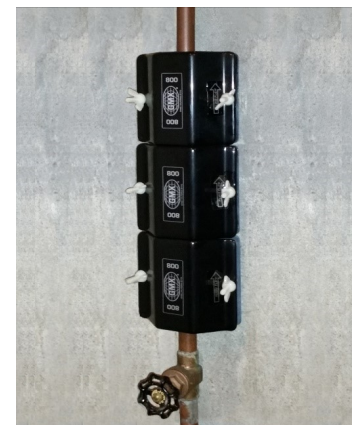
Water conditioners installed on the incoming waterline.
